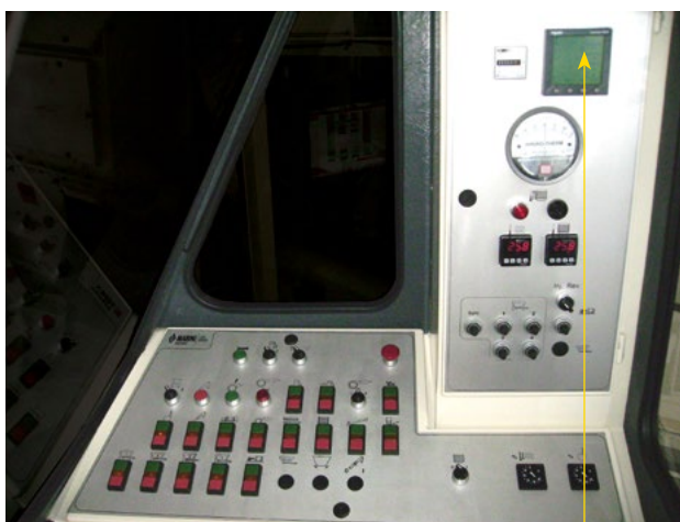
Painel de controle manual
